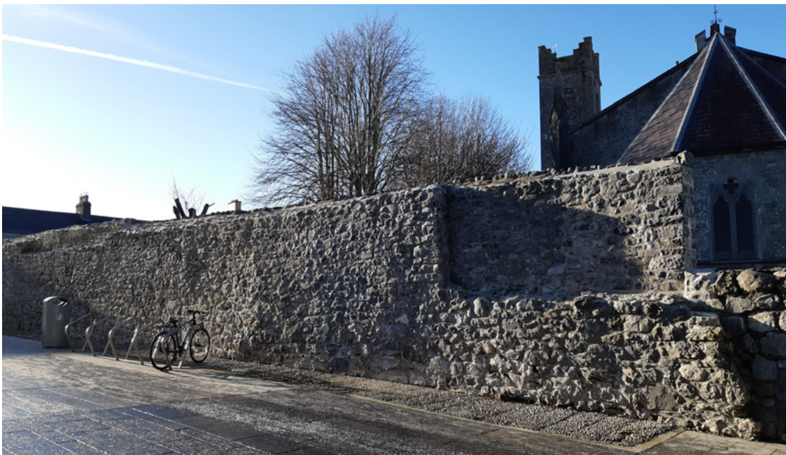
Athlone Town Wall at Church Street/St Mary's following conservation works funded by the Community Monuments Fund 2020 and 2021
